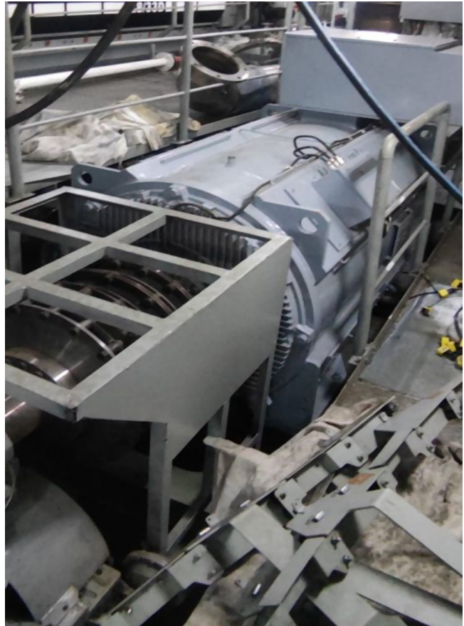
Fig. 4. Overview of a shaft generator in a ship.
